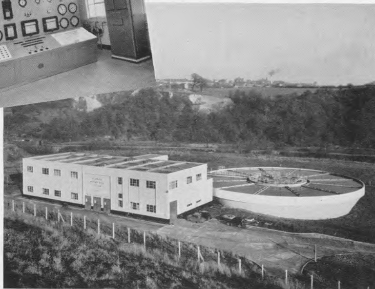
General view of water treatment plant—7½ million gallons a day
